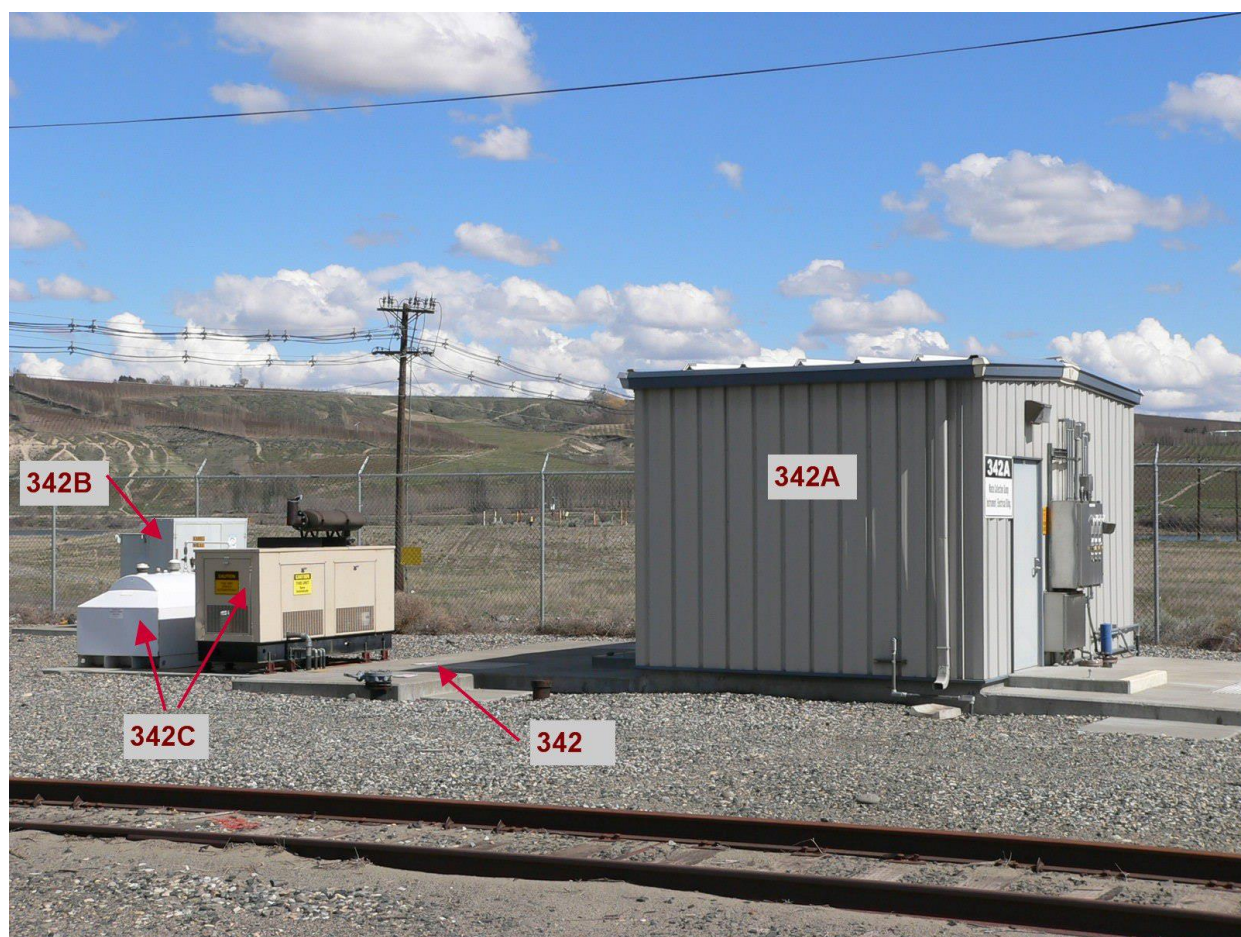
Figure 6. 342 Collection Sump (April 13, 2006).
