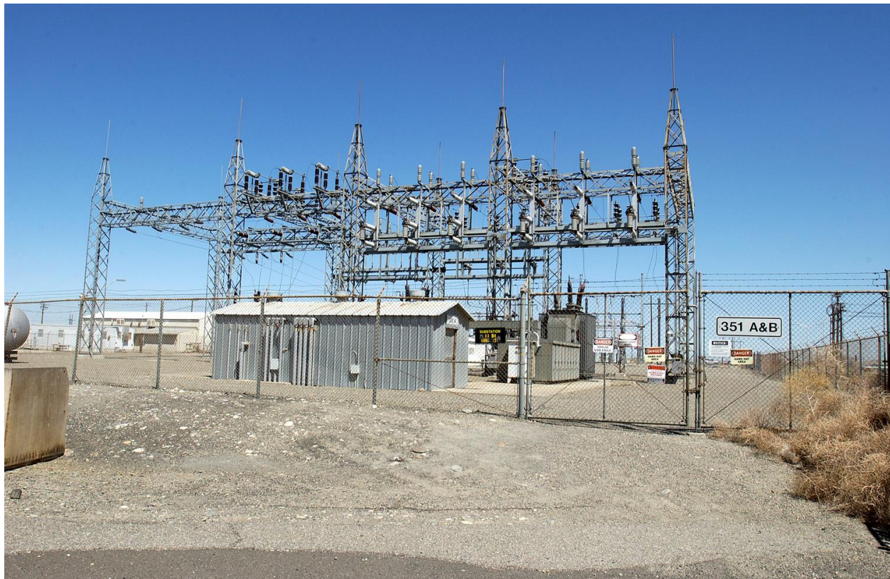
Figure 7. 351 Substation (B3S4) (June 30, 2003).
