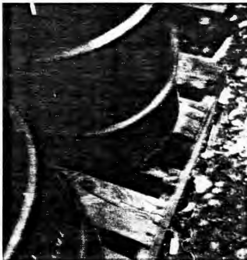
FIGURE 5. Photographs of Corroded Drums (Cont'd)
