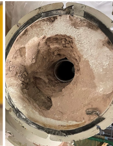
Outlet end of screw feeder
