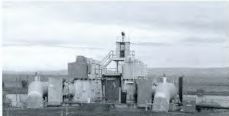
Pump controls and water lines that take water from the river to Hanford's Central Plateau. The new diesels provide backup power for pumps
