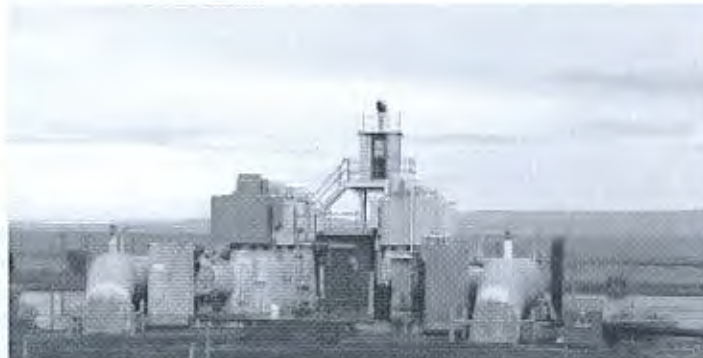
Pump controls and water lines that take water from the river to Hanford's Central Plateau. The new diesels provide backup power for pumps
