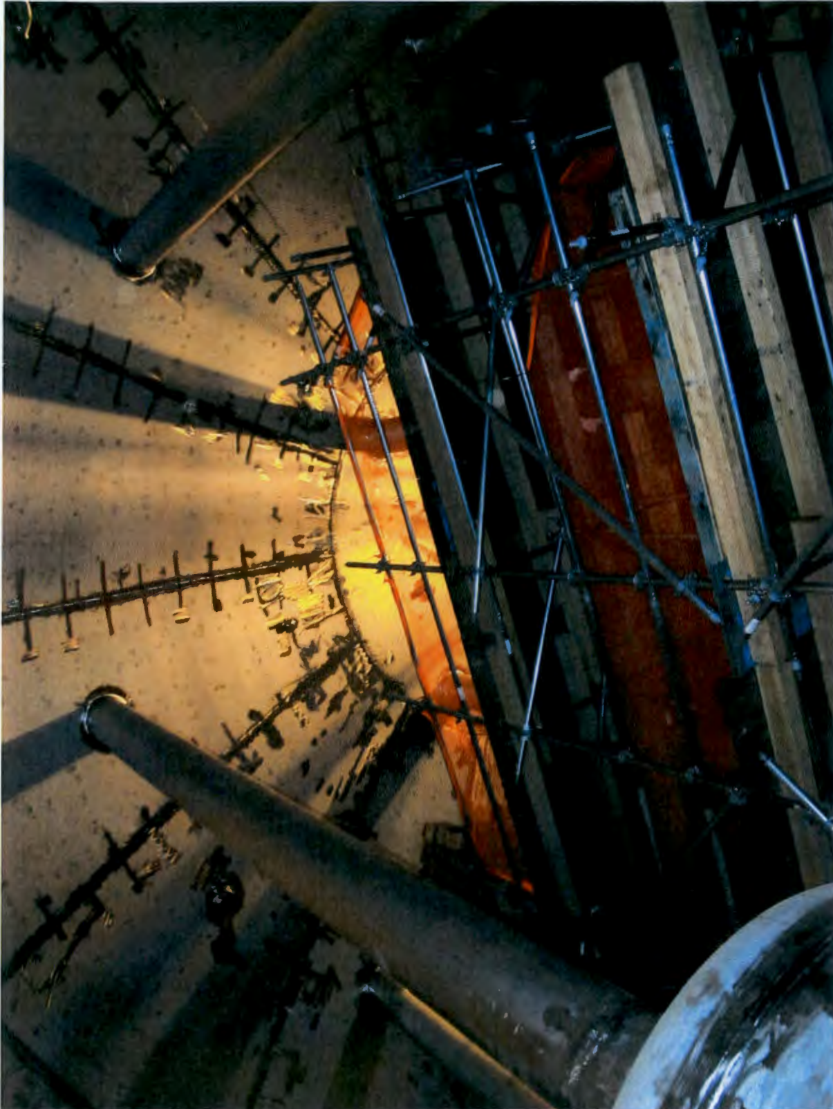
Figure 2 FRP-VSL-00002D Inside View
