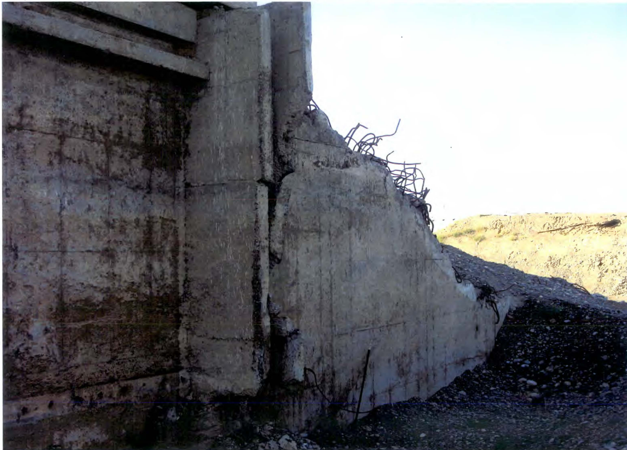
PHOTO # 148/109N W.Wall Below Grade SW Corner/EI.Varies/07-10-2012
