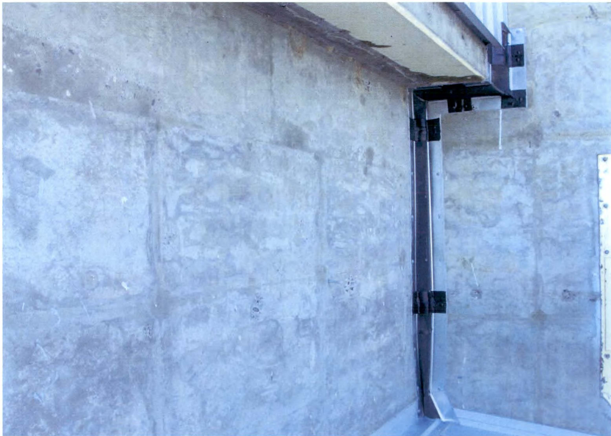
PHOTO # 120/109N/SSE Roof-Expansion Jt. Cover At Press./09-21-2011
