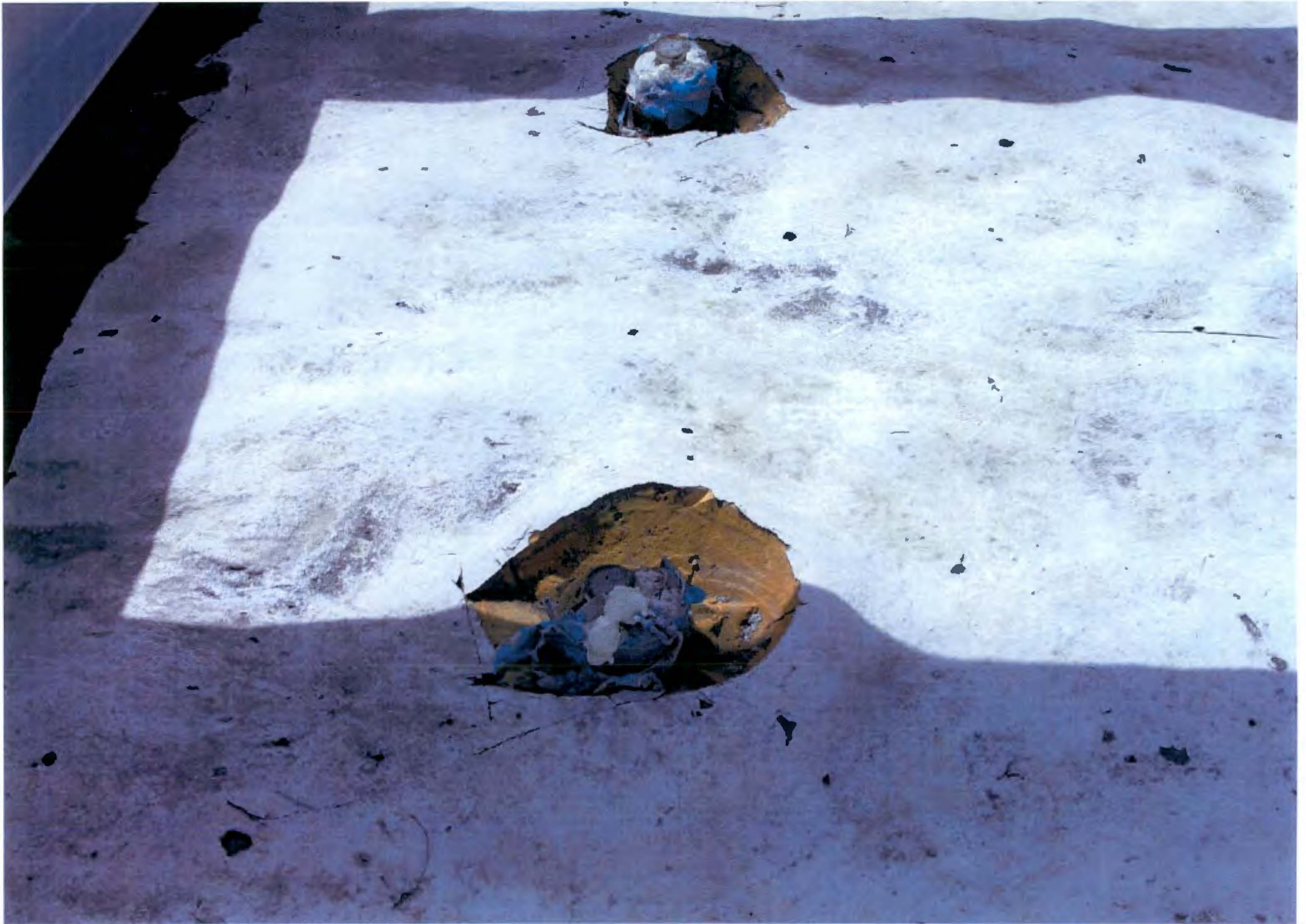
PHOTO # 125/109N Pressurizer/SSE Roof-Sealed Penetr./04-06-2011
