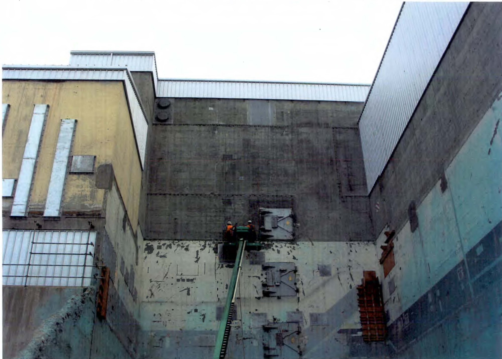
PHOTO # 545/105N/W.Wall Above Grade Between Rod Rm. & 109N/EI.Varies/07-19-2012
