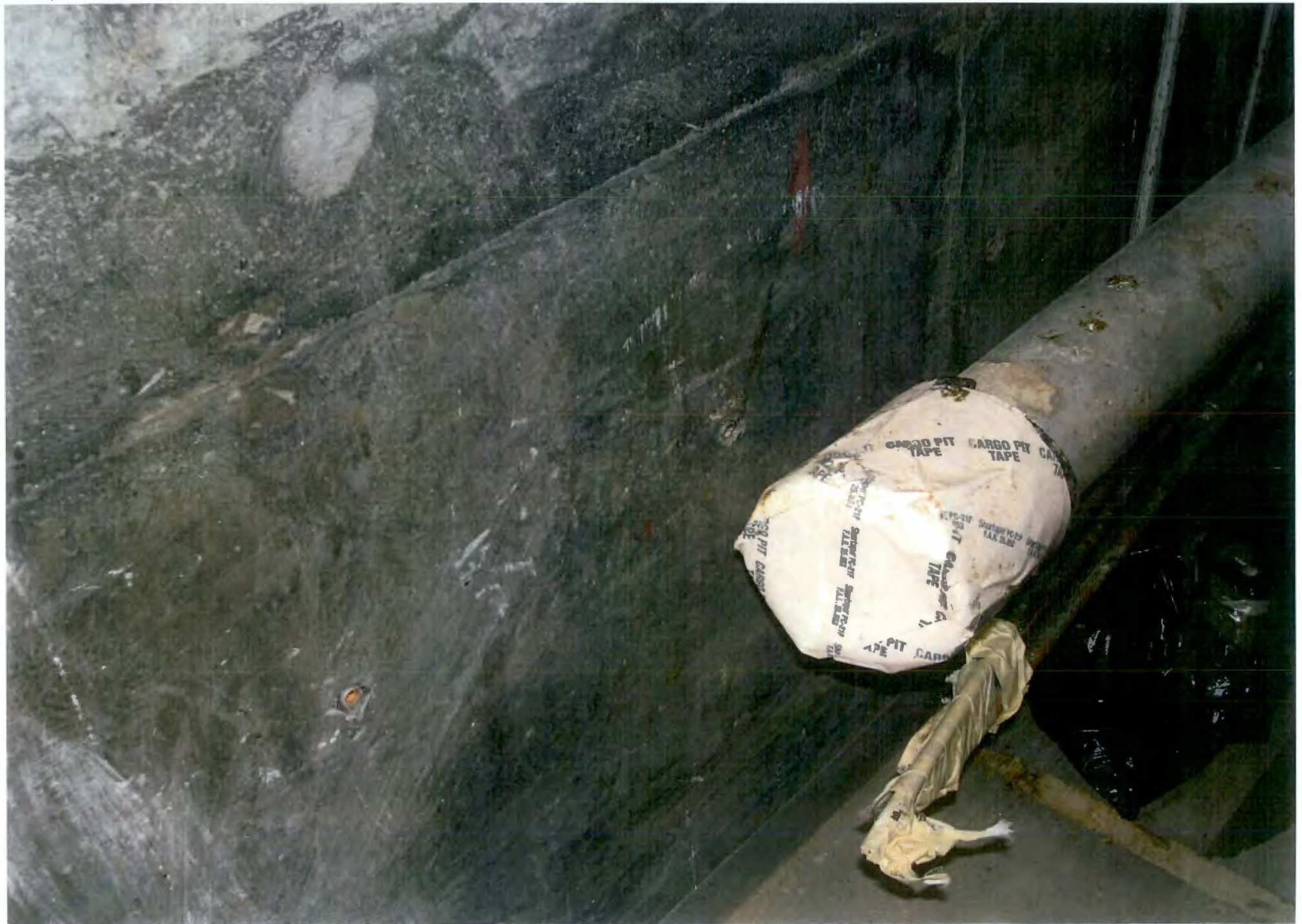
PHOTO # 530/105N/Corridor#7 FW Pipe at West End/EI.+5'-0"/06-05-2012
