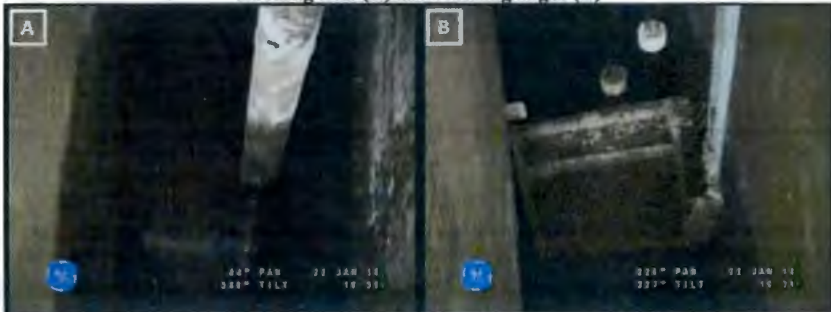
Figure 9. General Condition of the Annulus Floor on 1/22/2018 from Riser 89 Looking Left (A) and Looking Right (B)
