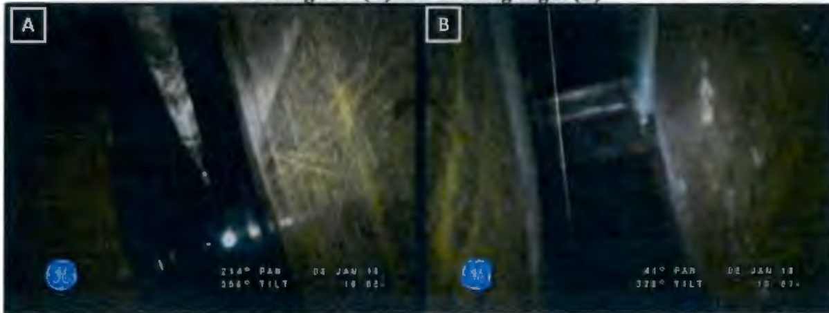
Figure 8. General Condition of the Annulus Floor on 1/8/2018 from Riser 88 Looking Left (A) and Looking Right (B)
