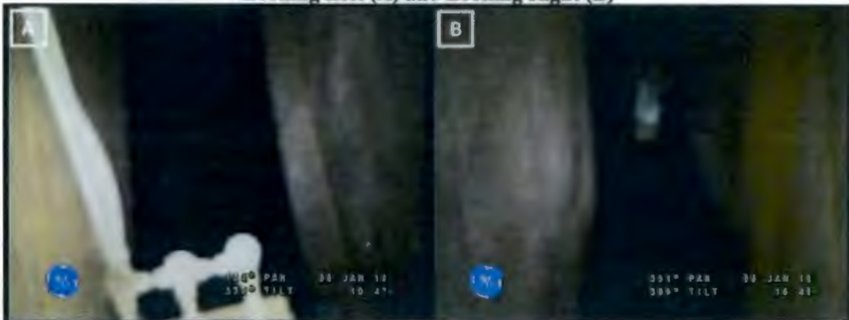
Figure 5. General Condition of the Annulus Floor on 1/8/2018 from Riser 80 Looking Left (A) and Looking Right (B)
