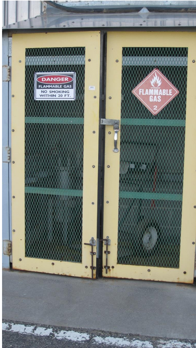
Figure 8. Flammable Gas Storage Area, 2734ZK
