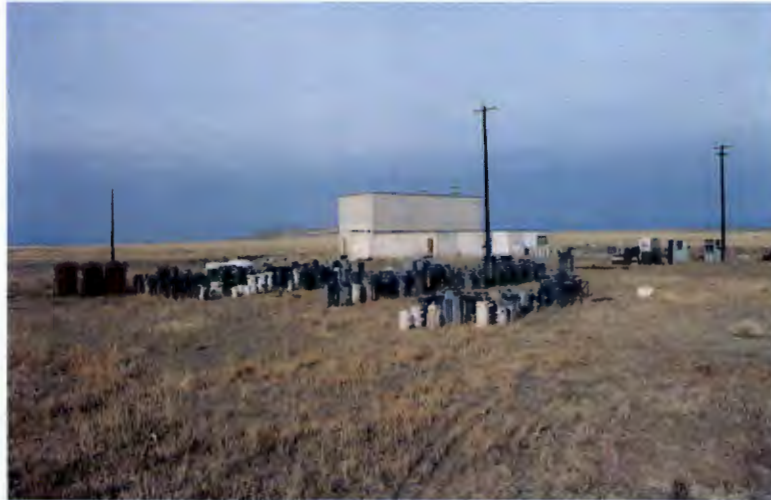
Figure 2-3. 212-P Facility with Outdoor Transformer Storage.
