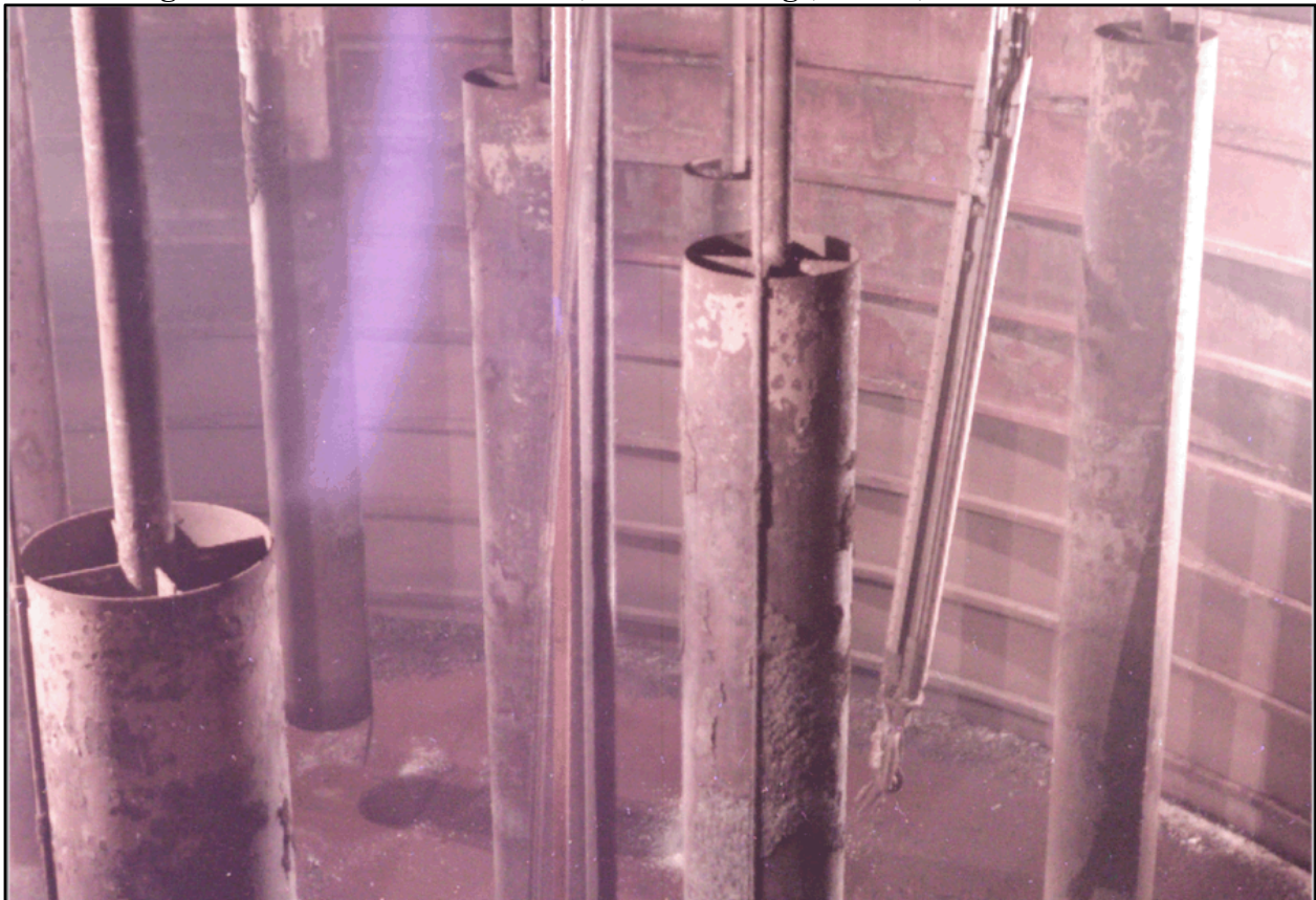
Figure 2-4. Waste on the Walls, Stiffener Rings, Risers, and Instruments.
